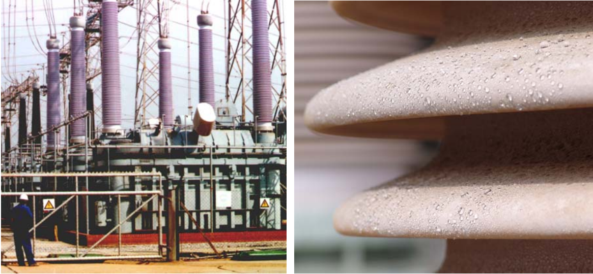
Figure 6: Coating condition at Apollo Converter Station after 8 years of service
